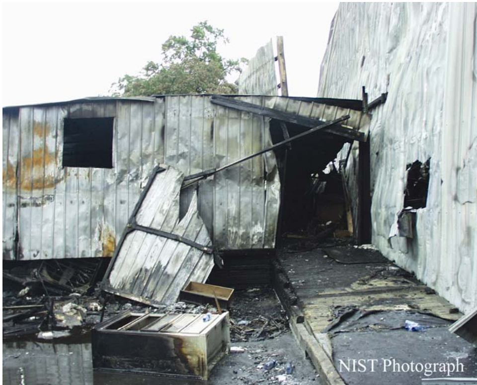
Figure 4-7. Photograph showing the outside of the loading dock. This was identified as the area of fire origin.
