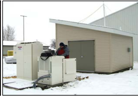
H 2 Generation & Storage
