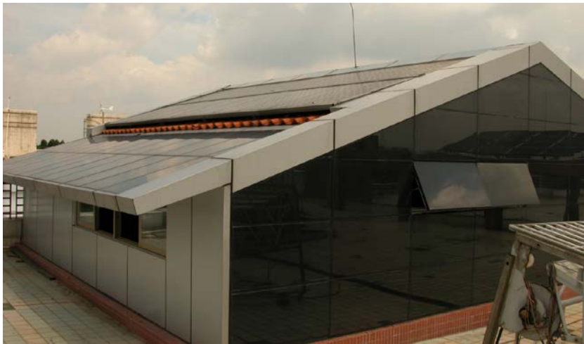
BIPV installation at SYSU (east campus)
