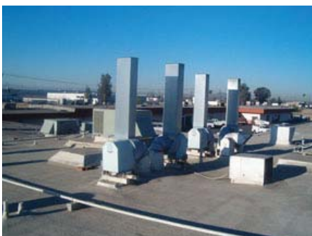
Laboratory Roof Fume hood Exhaust and Air Conditioning Systems
