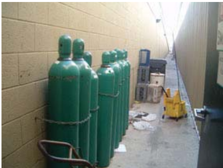
Laboratory Gases Cylinder Storage
