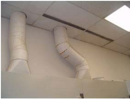
Laboratory Fume hood Unfiltered Make-up Air Intake Slots.
