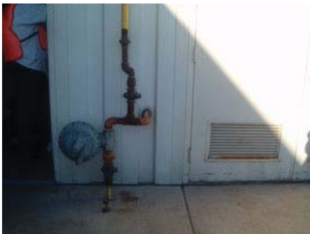
Natural Gas Service
