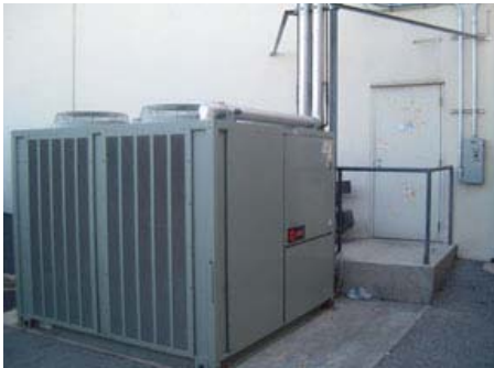
40 ton compressor unit
