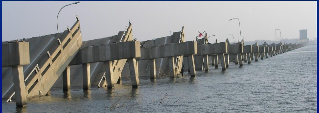
Bridge decks failure due to storm surge and wave action in Hurricane Katrina. Credit: NIST
