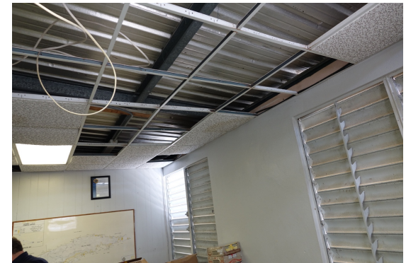
Damage to engineered building in Puerto Rico
