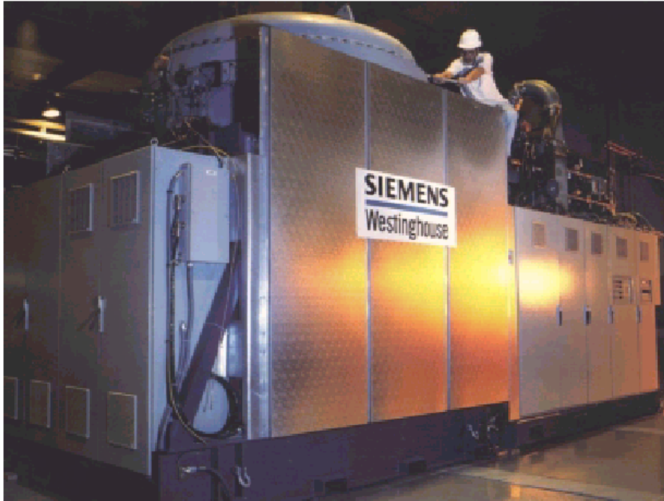
Figure 1. The SWPC 220 kW PSOFC/MTG
