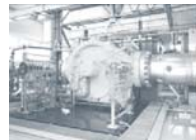
Small / medium centrifugal compressors
