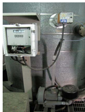
Waste incineration plants
