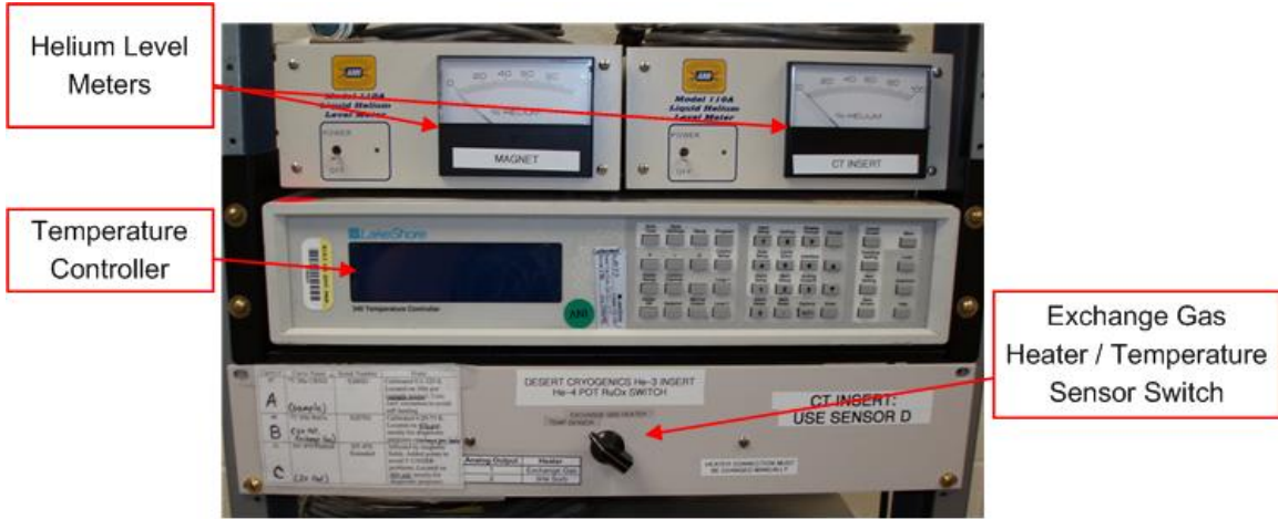
Figure 4: Electronics Rack Setup
