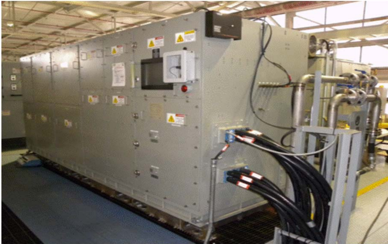
Existing 3 W 4160 VAC - 1000 VDC Power Conversion Module
