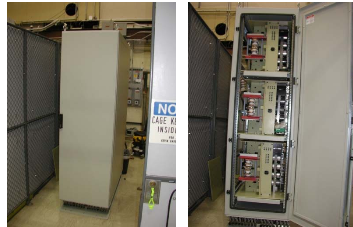
HPE - SSPS SiC 1 MW, 4160VAC-1000 VDC converter
