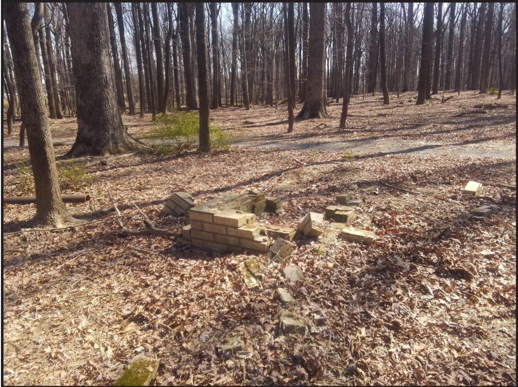
Figure 5.24 Collapsed brick chimney in Assessment Area 6
