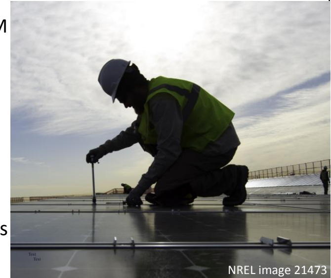
Cells can be cracked during installation
