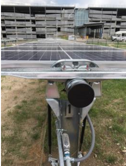
Field testing at NREL's small-scale outdoor test array
