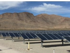
Field testing at two large-scale PV plants
