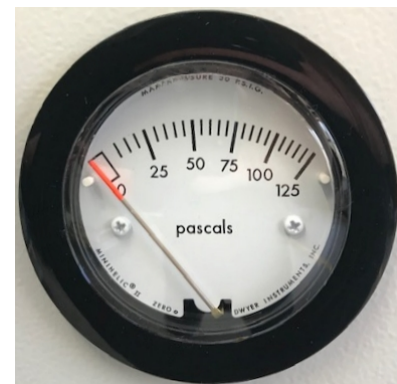
Figure 24: analog pressure display (manometer) for compressed air sweeping on the chamber front
