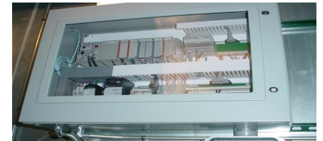
PLC and data acquisition system
