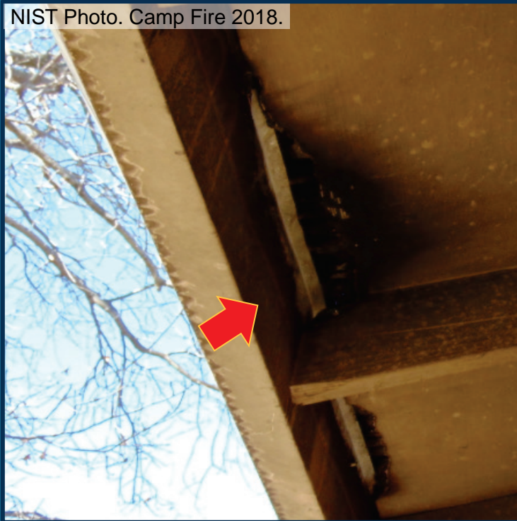
Failure: eave at fascia board
