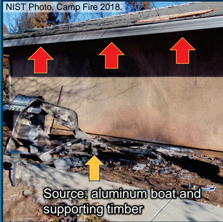
Failure: multiple locations along eaves
