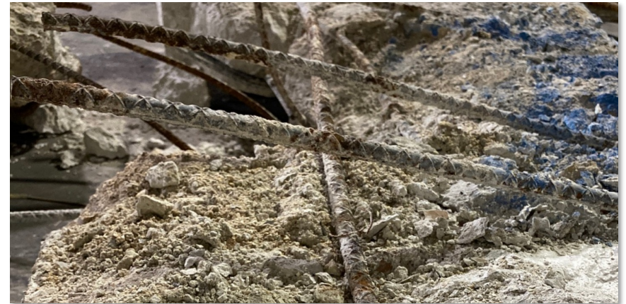
Measurement of degree of corrosion of steel reinforcing bars (assisted by NIST Statistical Engineering Division)
