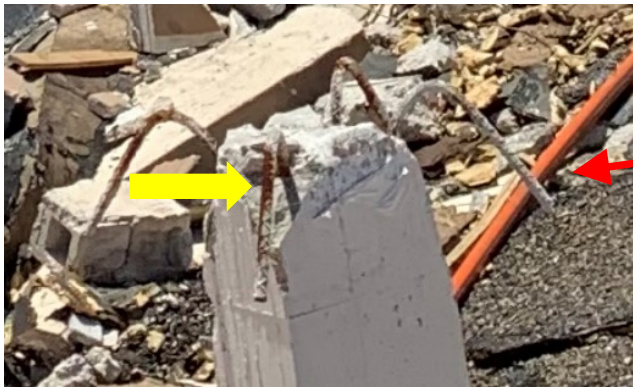
Enlargement of Column Top Showing Hooked Reinforcement Bars with Corrosion
