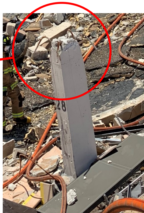
Pool Deck Column Post-Collapse
