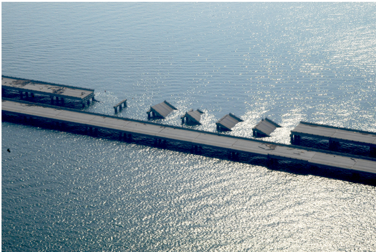
Figure 2: Bridge sections slid off their moorings during Hurricane Katrina.
