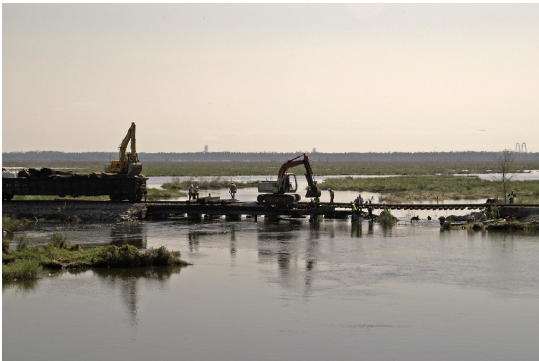
Figure 3: A railroad bridge in New Orleans is washed out by flooding.
