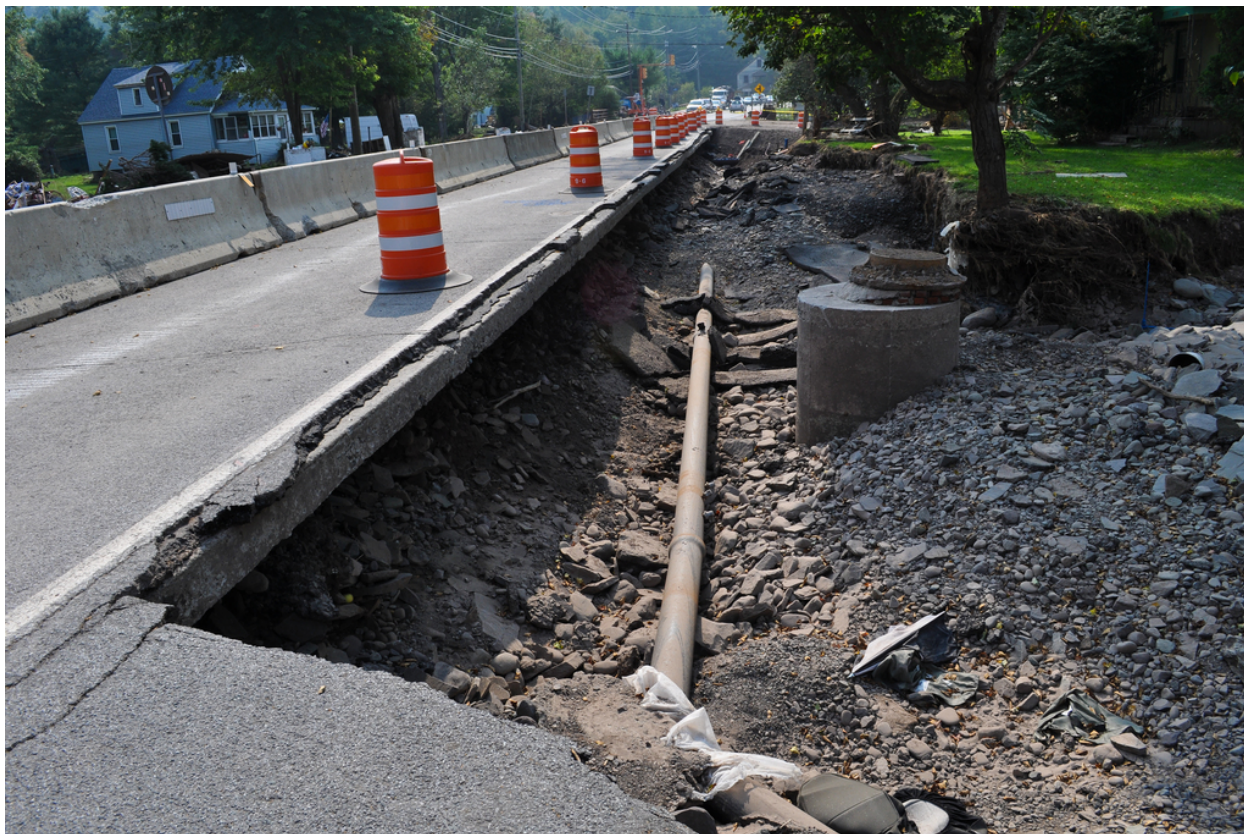
Figure 1: Road undercutting in the aftermath of Hurricane Irene.
