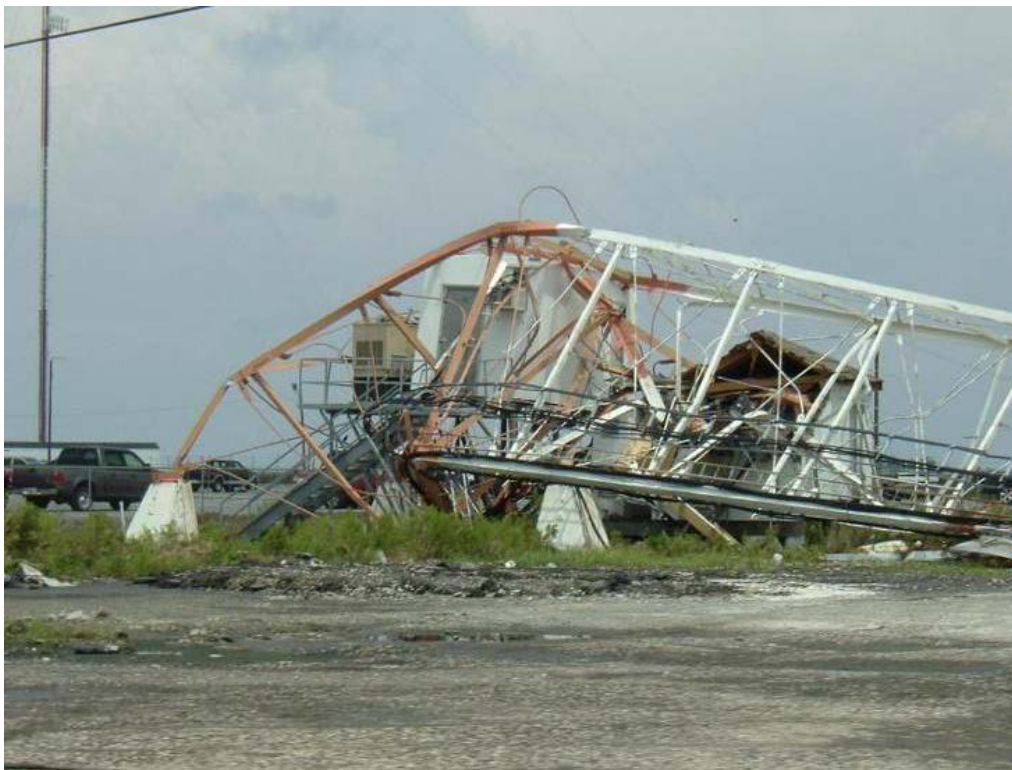
Figure 8-8. Tower Failed Due to Wind During Hurricane Katrina.
