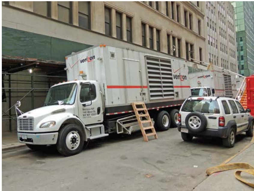
Figure 8-3. Large Standby Portable Power Unit used when Basement Generators Failed (FEMA 2013)
