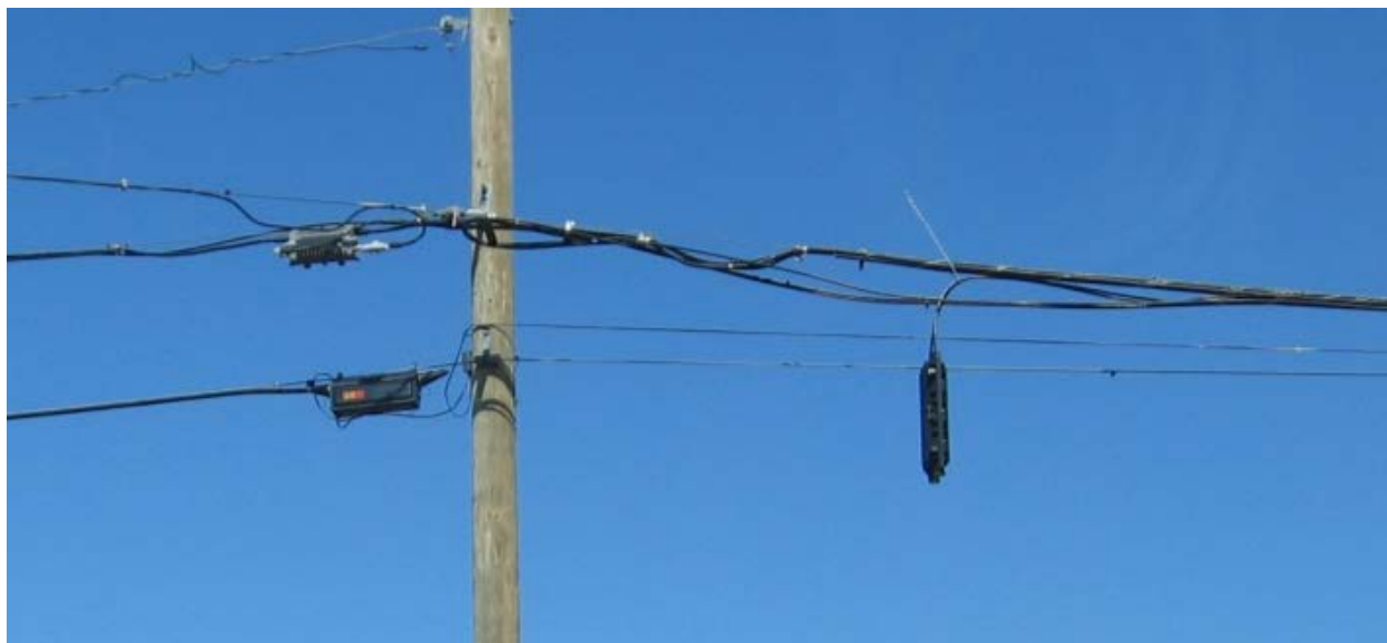
Figure 8-5. Failure of CATV cable due to the direct action of wind.
