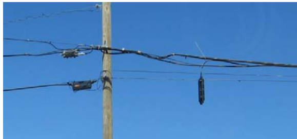
Figure 8-6. Failure of CATV cable due to the direct action of wind (Kwasinski 2006)
