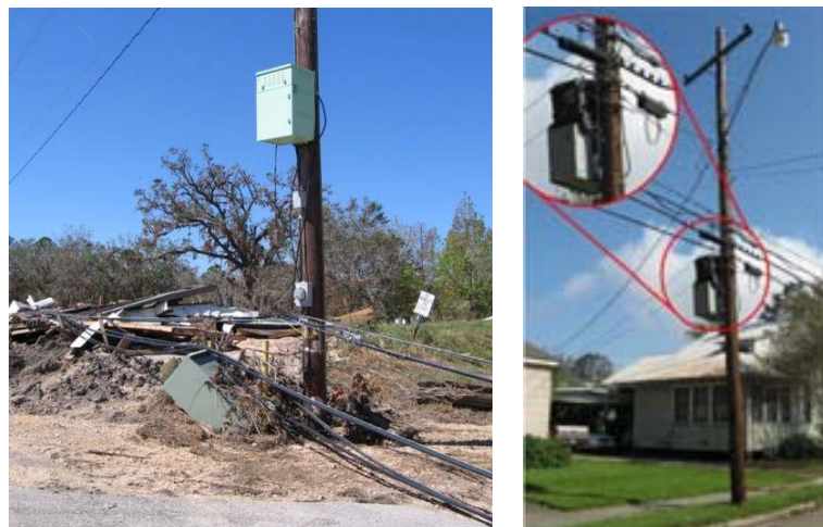
Figure 8-9. Placement of UPS Systems is an Important Consideration for Resilience and Periodic Maintenance (Kwasinski 2009)
