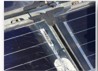
G/G modules cracking at clamps due to local strain 1.5 years, NW China
