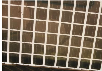
Severe delamination on glass/glass module 10 years, Arizona USA
