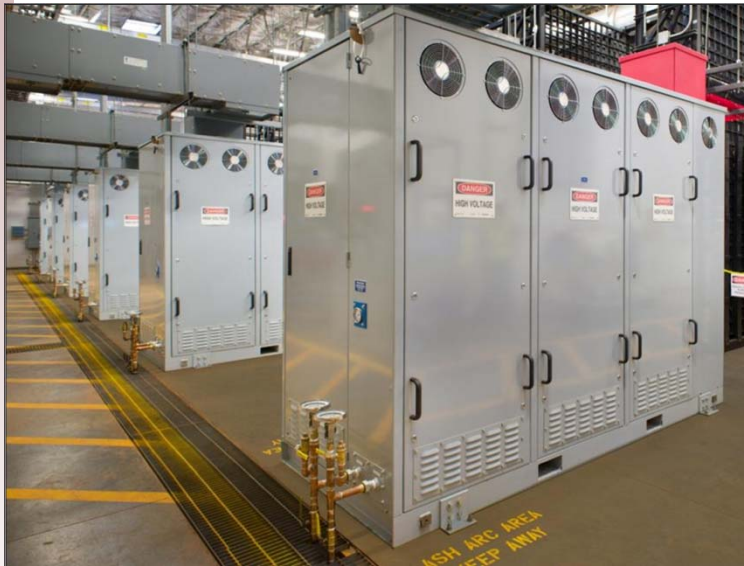
1.5MW Inverters installed at Xtreme Power BESS in Hawaii
