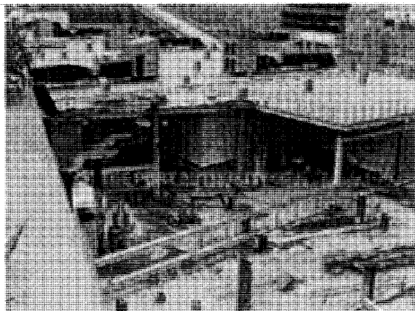
Figure 68. Infected beams removed, probably within days. (6/?/06) Source:
