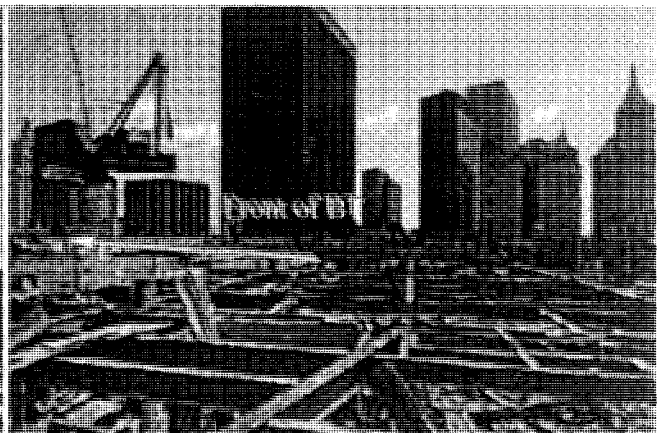
Figure 64. Once the concrete slab and metal decking are removed, what remains is a steel skeleton of each floor. There is little rust in the southwest corner of the building, even though it is open during the deconstruction from the top down. 17bank_CA06.jpg
