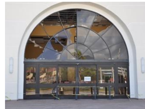
Windows with Broken Glass
