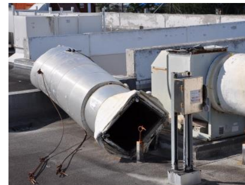
Damaged/Dislodged Rooftop Equipment
