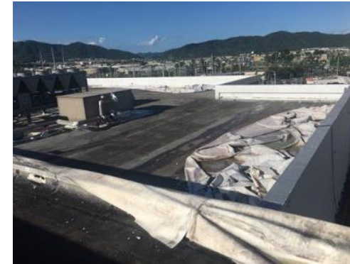
Damaged Roof Covering
