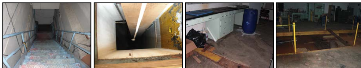
FIGURE 25: The Underground Silo Reconnaissance task included negotiating and inspecting a defunct underground Nike missile silo with multiple complex rooms, uneven flooring obstacles, and extensive radio attenuation. Entry could be gained by A) descending a stairway with 40 degree incline and 9 inch risers or B) vertical insertion through a manhole ladder. C) Barrels with four directional targets to identify were placed throughout the environment requiring access to confined areas to identify targets from all directions. D) A variety of flooring complexity divided the space. Two different operator stand-off positions were available depending on radio communications capability of the robot: 10m (top of the stairs), 100m non-line-of-sight.
