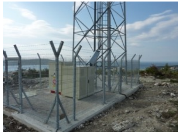
Figure 8-7. Base of Cell Tower Showing Standby Power and Switch Gear
