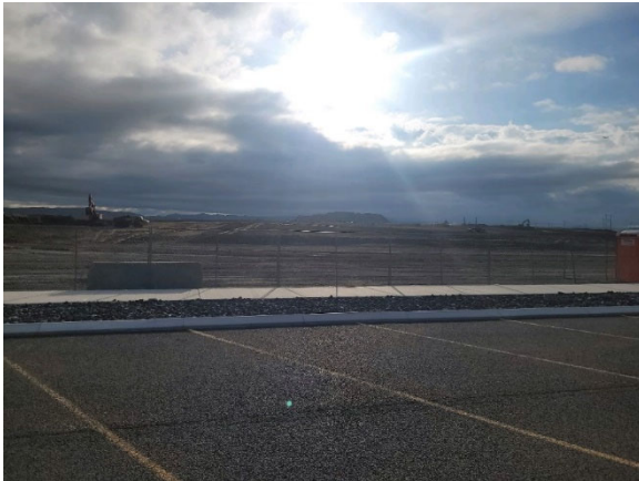
Figure 9. Ongoing Cut and Fill Excavations within the APE near the Micron Campus.
