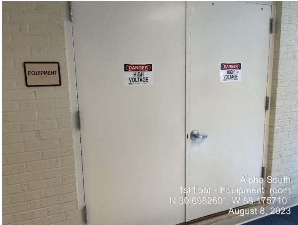
Photograph 19 – Alpha South – Electrical Equipment Room.
