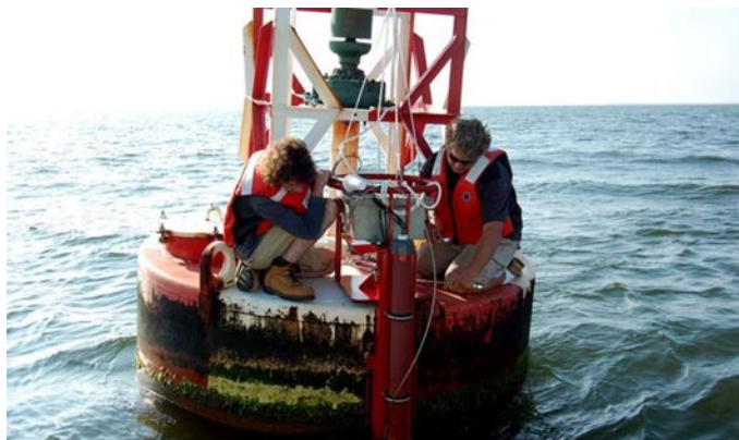
Max Ivanov and Scott Mowery with NOAA's Center for Operational Oceanographic Products and Services install an improved current sensor system on a navigation buoy in Chesapeake Bay. The system transmits real-time current speed and direction observations via satellite to help mariners more safely navigate busy shipping channels. (Photo: NOAA)
