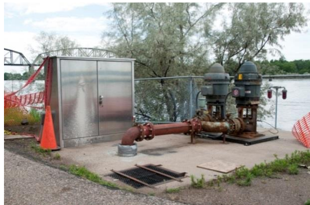
Figure 9-5. Bismarck, ND Pump Station Damaged by Flood Inundation from Adjacent Missouri River (Courtesy of FEMA)
