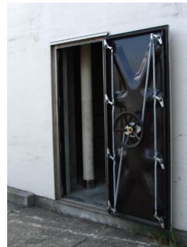
Figure 8-4. Watertight Door Used on Central Office in Kamaishi, Japan (Kwasinski 2011)
