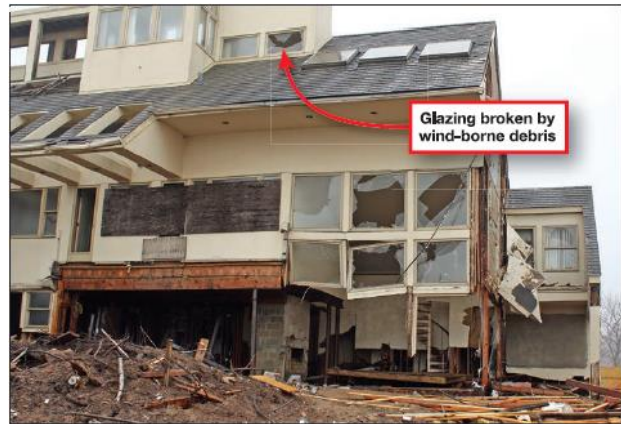
Figure 5-11: Wind and wind-borne debris resulted in considerable damage to glazing on this building (courtesy of FEMA) [getting a better quality version]
