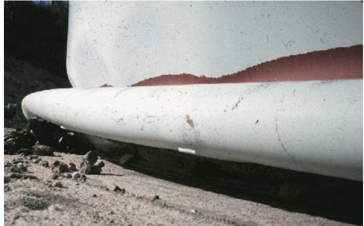
Figure 9-9. Steel Tank “Elephant’s Foot” Buckling in 1994 Northridge Earthquake (Courtesy of Donald Ballantyne)
