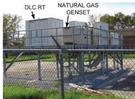
Figure 8-8. Elevated DLC RT with Natural Gas Standby Generator Installed After Hurricane Katrina (Kwasinski 2011)
