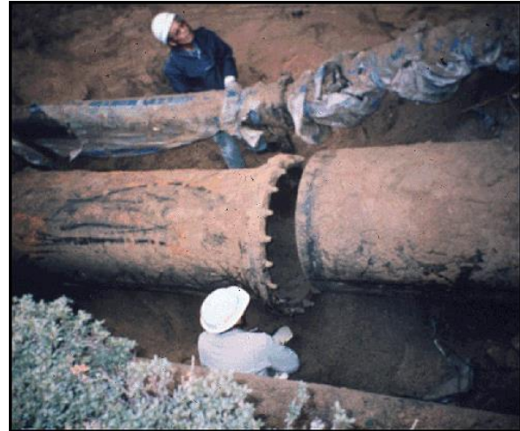
Figure 9-11. Joint Separation in Ductile Iron Pipe due to Liquefaction during 1995 Kobe Earthquake (Courtesy of Kobe Water Department)
