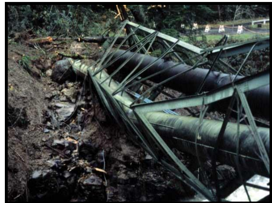
Figure 9-2. Water Transmission Pipeline Bridge Damaged by Landslide (Courtesy of Portland Water Bureau)
