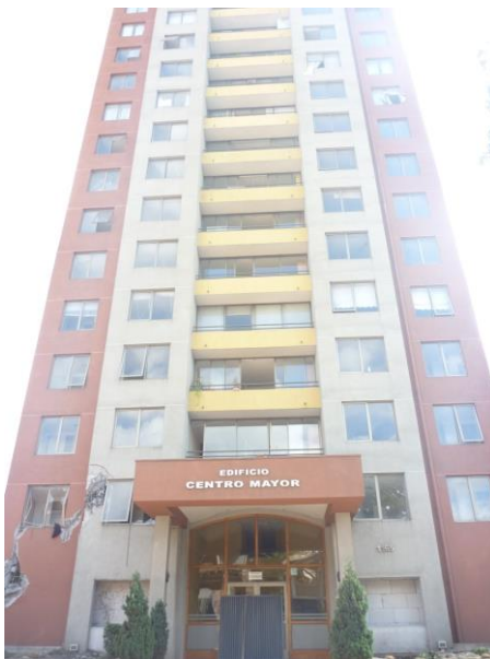
Figure 5-8: Apartment building with damaged structural members that is globally stable. (courtesy of Degenkolb Engineers)
