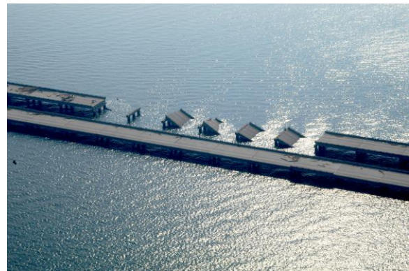
Figure 6-3: Bridge sections slid off their supports during Hurricane Katrina due to wave action (FEMA, 2005)
