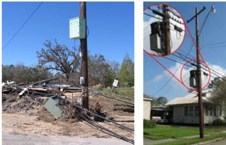
591 Figure 8-9. Placement of UPS Systems is an Important 592 Consideration for Resilience and Periodic Maintenance 593 (Kwasinski 2009)
