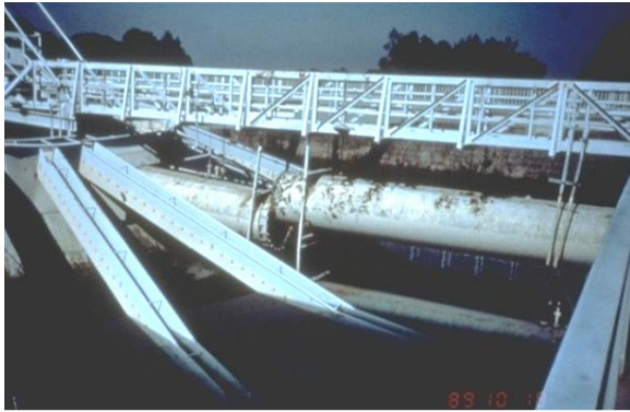
Figure 9-3. Santa Clara Valley Water District, Rinconada Water Treatment Plant Clarifier Launderers Damaged due to Sloshing, 1989 Loma Prieta Earthquake (Courtesy of Don Ballantyne)
