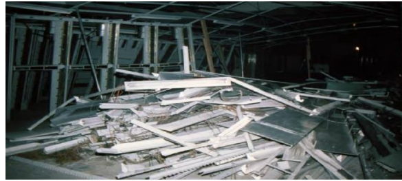
Figure 8-5. Light Fixture and Equipment Failure inside Central Office in Mexico City 1985 Earthquake (Alex Tang, OSSPAC 2013)
