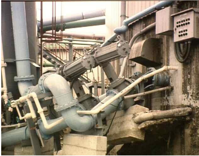
Figure 9-12. Non-Pile Supported Structures Failed Due to Liquefaction in 1995 Kobe Earthquake (Courtesy of Donald Ballantyne)
