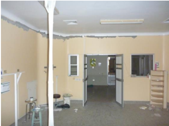
Figure 5-2: Non-structural damage to interior finishes following an earthquake event. (Photo Courtesy of Degenkolb Engineers)
