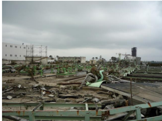
Figure 9-15. Sendai WWTP Equipment and Piping Damage from 2011 Earthquake (Courtesy of Donald Ballantyne)
