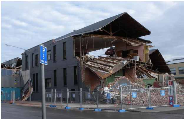
Figure 5-1: Failure of unreinforced masonry wall during an earthquake event. (Photo courtesy of Degenkolb Engineers)
