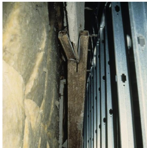
Figure 5-9: Fractured brace connection in a building damaged in an earthquake (courtesy of Degenkolb Engineers)
