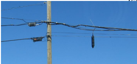
452 and ice hazards. In high wind events, overhead wires 453 may fail due to the failure of poles by the direct 454 action of wind acting on poles and cables, or trees 455 falling onto the cables. Figure 8-6 shows an example 456 of a failed cable television (CATV) line due to the 457 direct action of wind during Hurricane Katrina. Figure 8-6. Failure of CATV cable due to the direct action of wind (Kwasinski 2006)
