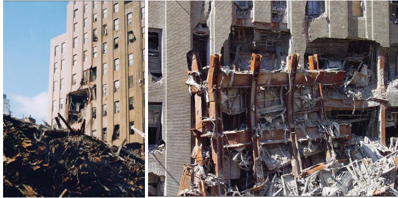
Figure 8-2. Damage to Verizon Building on September 11, 2001 (FEMA 2002)
