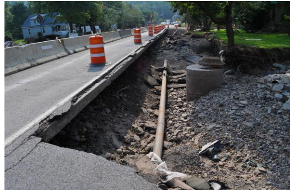
Figure 6-1: Road undercutting in the aftermath of Hurricane Irene (FEMA, Photo by Elissa Jun, 2011)
