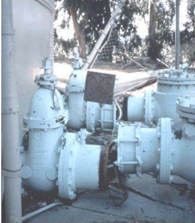
Figure 9-8. Tank Moved, Severing Connecting Pipe in 1994 Northridge Earthquake (Courtesy of Los Angeles Department of Water and Power)
