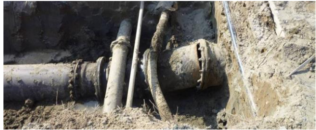
Figure 9-4. Liquefaction Caused Differential Settlement Between Pile-Supported Structures and Buried Pipe during the 2011 Tohoku Earthquake (Courtesy of Don Ballantyne)
