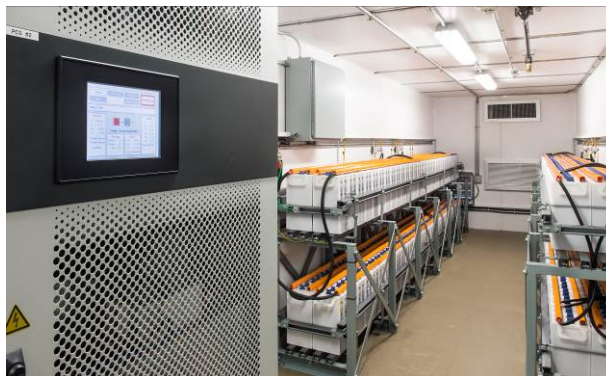
An example of a stationary, grid-connected battery is the NREL project from Erigo/EaglePicher Technologies, LLC Technologies.
