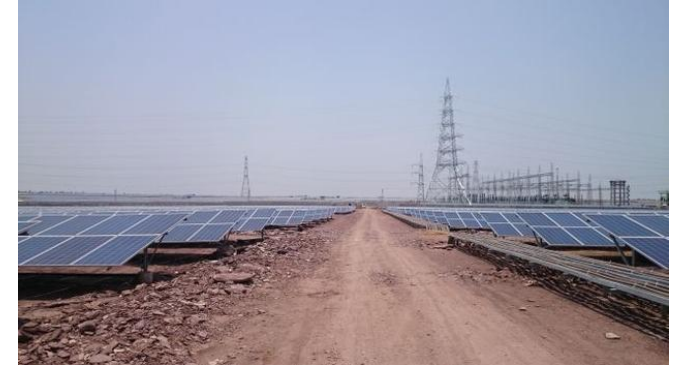
Kurnool Ultra Mega Solar Park, 900 MW, India
