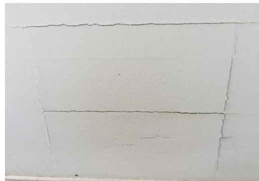
Cracking in PA Backsheet
