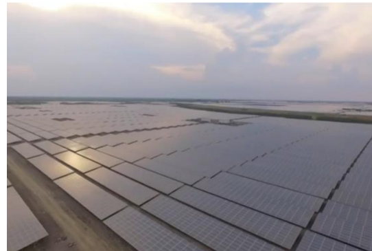
Kamuthi Solar Power Project, 648MW, India
