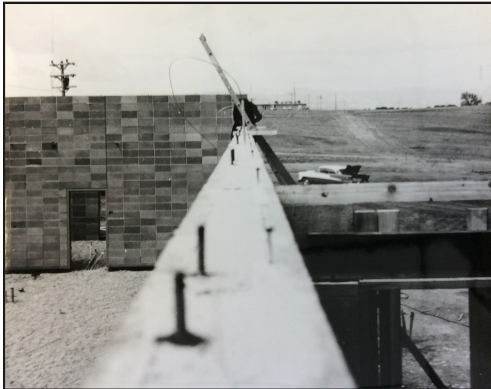
Figure 3.2: Construction of Radio Station WWV at Fort Collins, Colorado, 1966 (courtesy of NIST Fort Collins).
