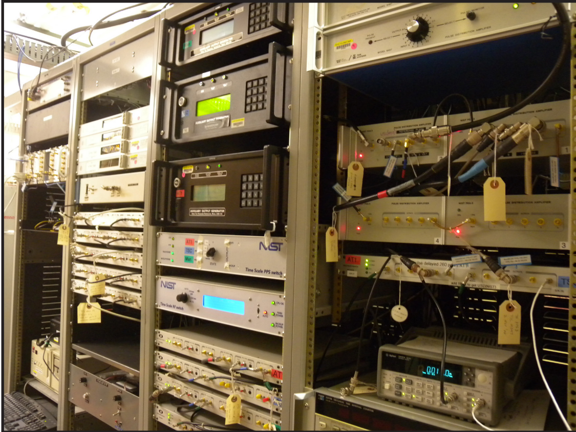
Figure 1.3: Mechanical Room Equipment for the Cesium Atomic Clock at Building 1 of Boulder Laboratories in Colorado.
