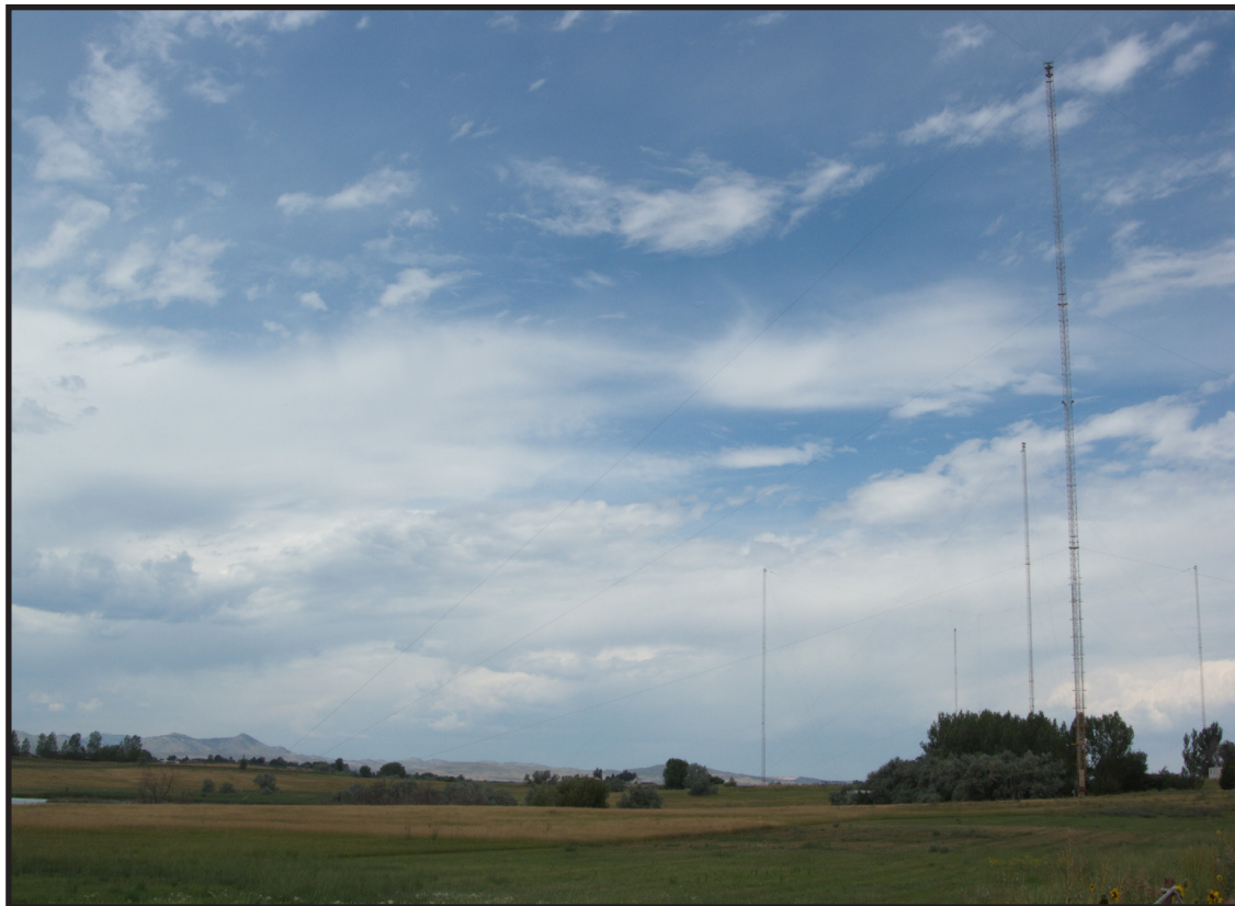
Figure 4.6: WWV Antenna Systems at Fort Collins, Colorado, facing southeast. August 2019.
