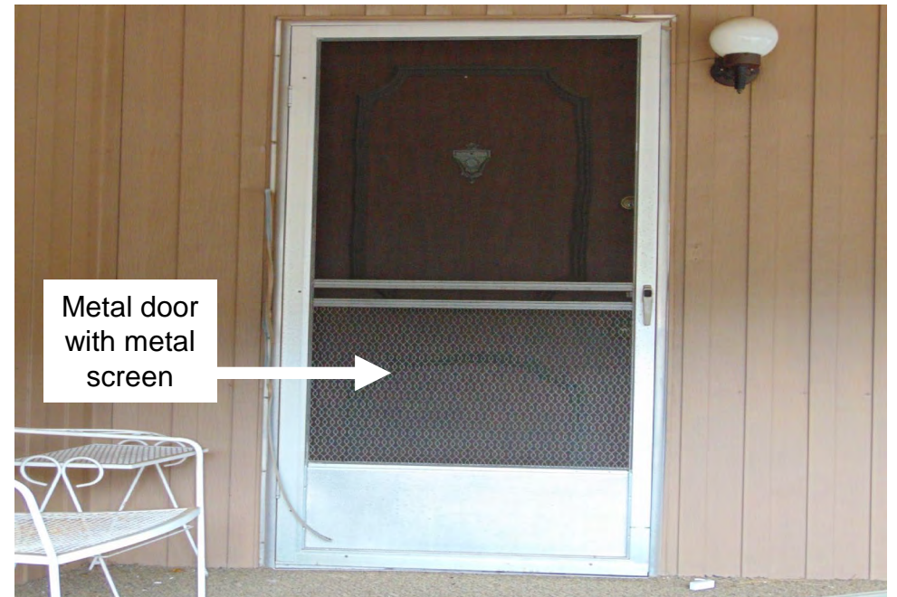
Item 26 Plastic Screen Door – Replace plastic screen doors with metal screens and doors to reduce ignition risk.
