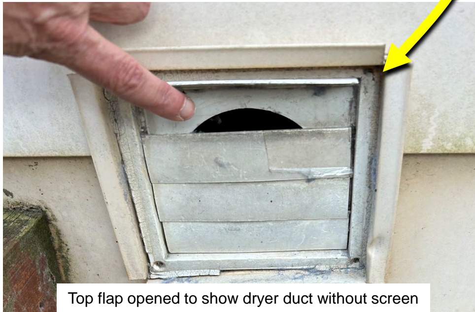
Plastic cover for dryer vent without fine metal mesh screen
