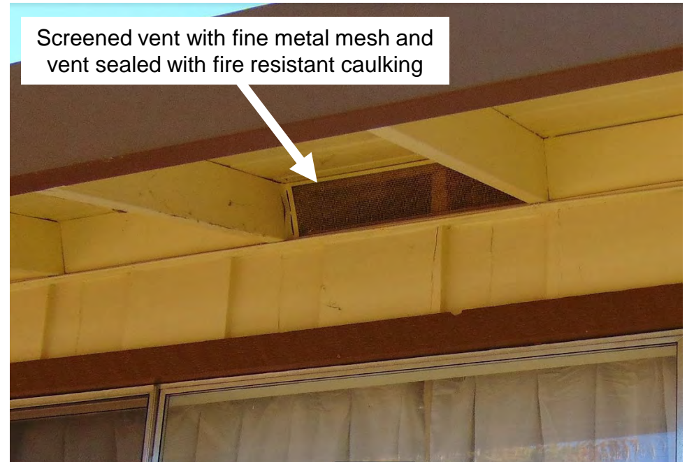
Item 14.1 Under Eave Vent (Vertical) – Keep vents clean, cover with a 1/8 th inch fine metal mesh screen, and seal vent with fire-resistant caulking.
