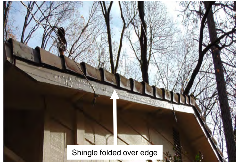
Item 8.3 & 9 No Gutters – Roof edge without gutters can leave combustible roof materials exposed.
