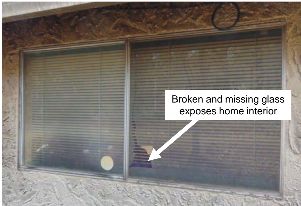
Item 22 Window (Single Pane) – Replace with non-combustible frame and double pane tempered glass window.
