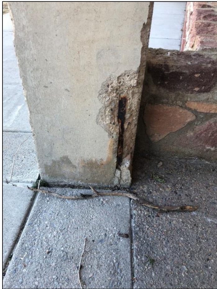
Photo C-154. Spalls at Steel Embed
