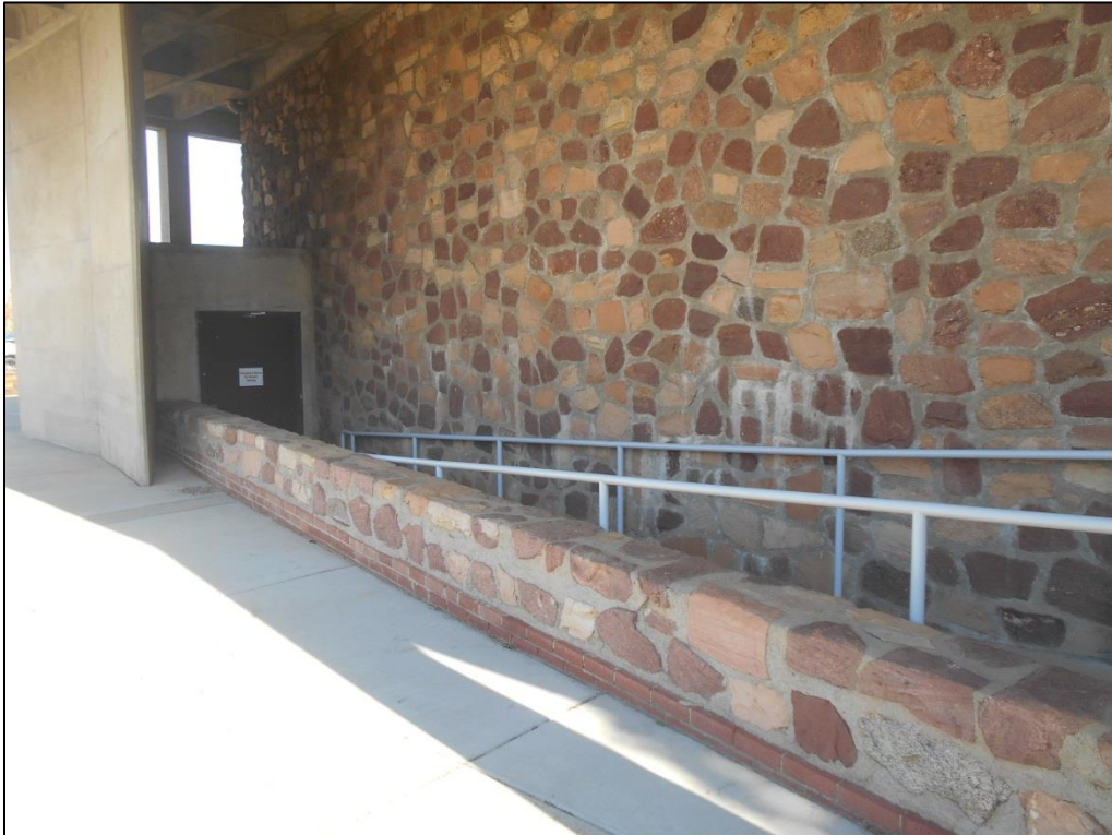
Figure C-6. Ramp to West Auditorium Stage Door, Stone and Brick Retaining Wall, and "Butterfly" Screen Wall (view northeast)
