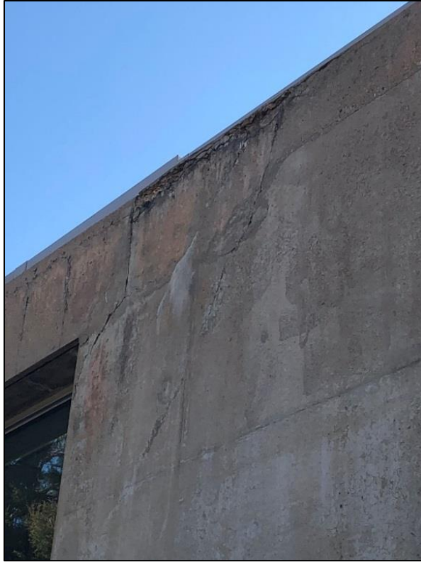
Photo C-155. Water Exposure and Cracks
