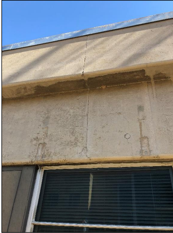
Photo C-161. Cracks in Roof Beam
