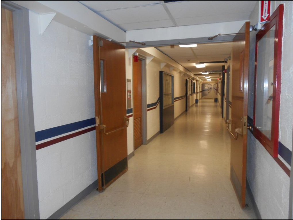
Photo C-127. Double Loaded Corridor in Level 2 of the Spine, South of the Intersection of Wings 1 and 2 (view southwest)
