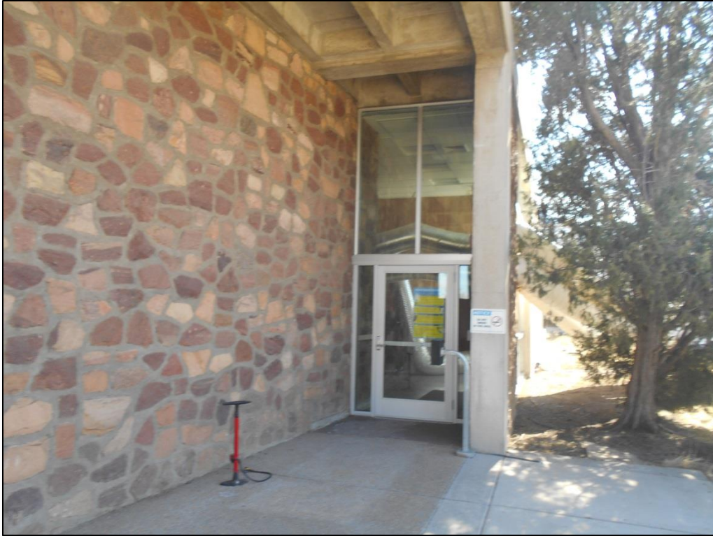
Figure C-5. North-Facing Exterior Door on the West Side of the Auditorium (view southwest). This door was replaced in 1981.
