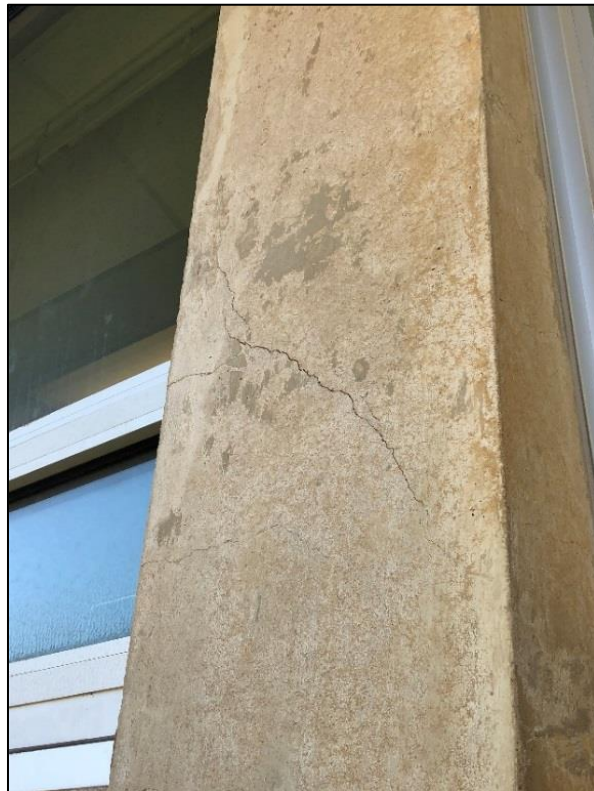
Photo C-158. Column Cracks and Stains
