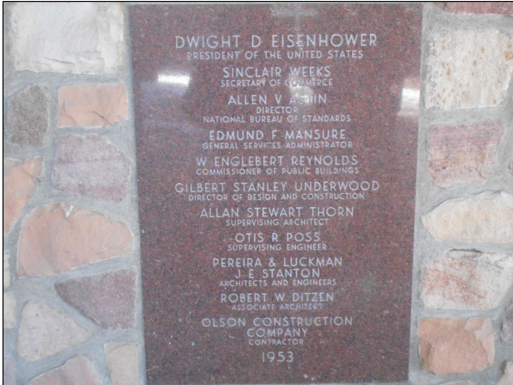
Photo C-117. Cornerstone Monument on the East Exterior Wall of the Auditorium (view northwest)
