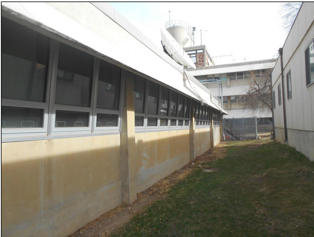
Photo C-34. Orange Staining on Concrete and Replacement Windows on North Elevation of Wing 1 (view southeast)
