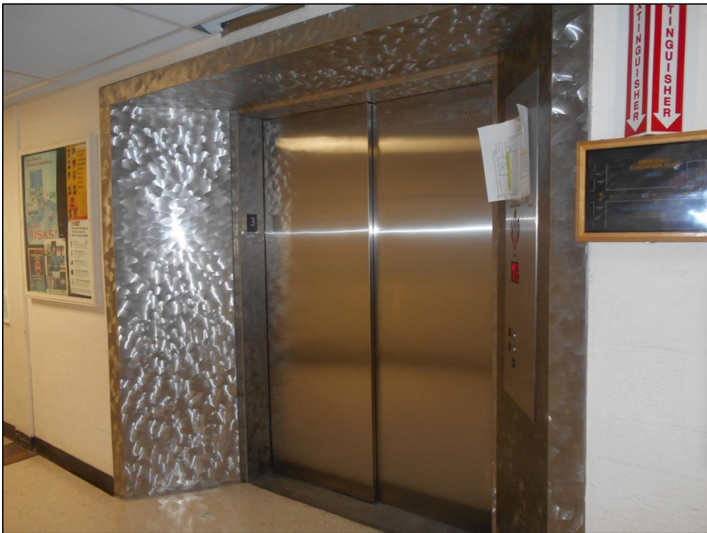
Photo C-138. Upgraded Elevator in Level 3 of the Spine
