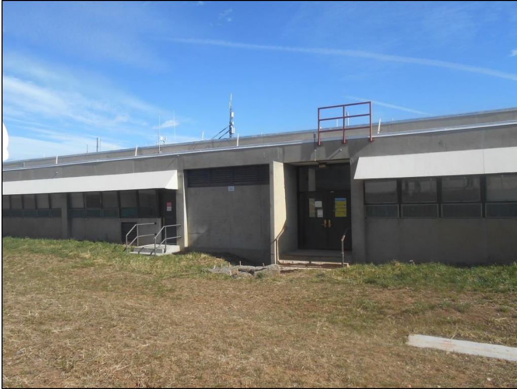
Photo C-61. Doors on South Elevation (view north); the single-leaf door on the left is a later addition and is not an original feature of Wing 2
