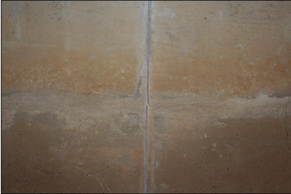
Photo C-49. Concrete Wall Detail with Horizontal Pour Line, Vertical Control Joint, and Orange Concrete Stains; Typical of Wings 1, 2, and 4.
