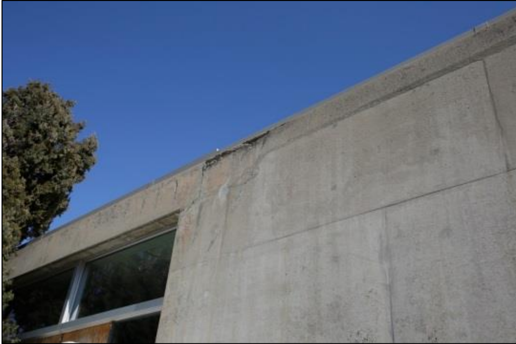
Figure C-3. Concrete Spalling on West Elevation of Auditorium
