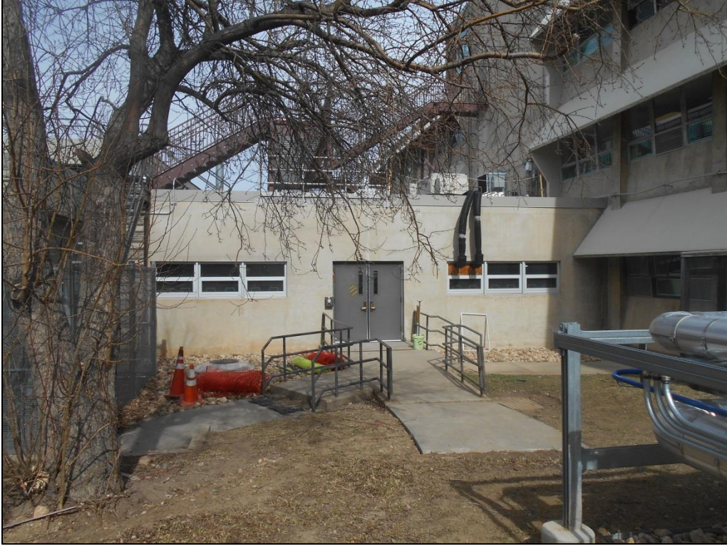
Photo C-37. Replacement Windows and Original Door on South Elevation of Wing 1 Hyphen (view north)
