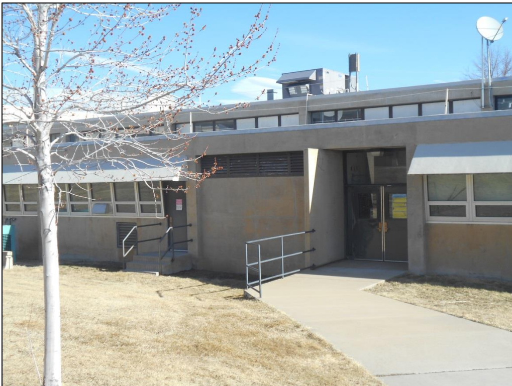
Photo C-52. Doors on South Elevation of Wing 2 (view north); the single-leaf door on the left is a later addition and is not an original feature of Wing 2
