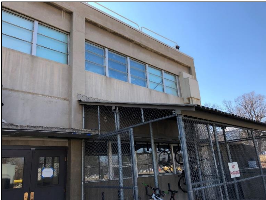
Photo C-164. Deterioration of Existing Canopy
