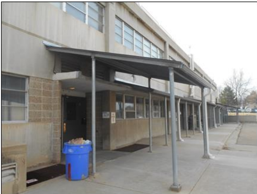
Photo C-68. Failed Original Concrete Canopy and Metal Awnings on North Elevation (view west)
