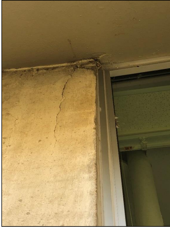
Photo C-159. Cracking at Top of Column
