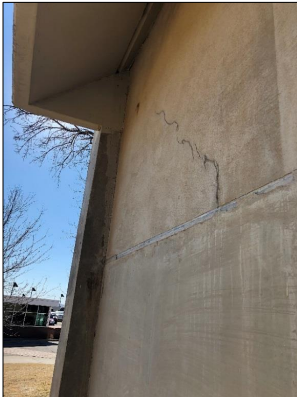
Photo C-160. Cracks in Wall
