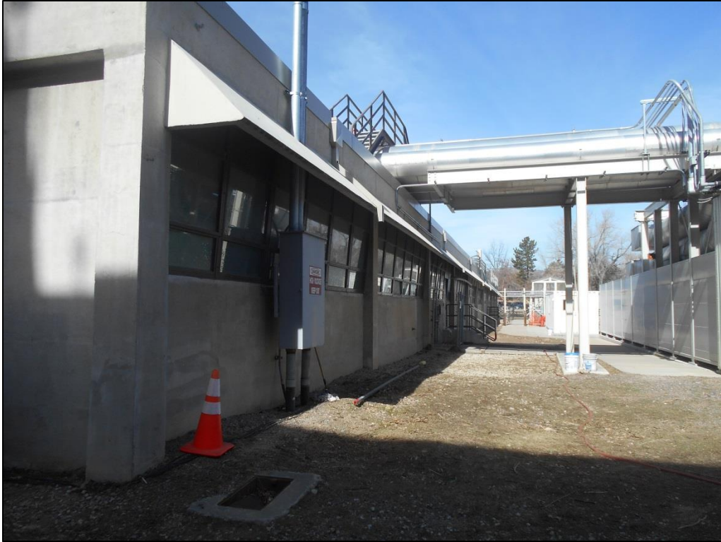
Photo C-45. Connections between Annexes D and E to the Rooftop of Wing 1 (view northwest)
