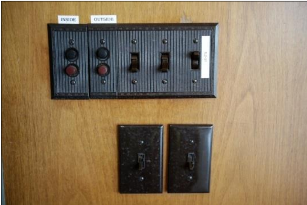
Photo C-110 Electrical Switches in the Reception Area
