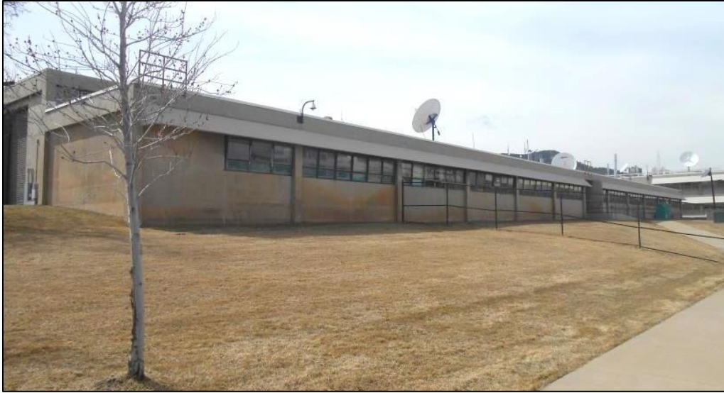
Photo C-63. East Elevation of Wing 4 (view west); three original windows have been removed from the first bay
