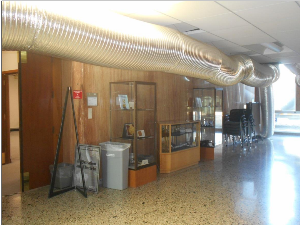
Photo C-95. South Wall of the Foyer between the Entrances to the Lecture Rooms (view west)
