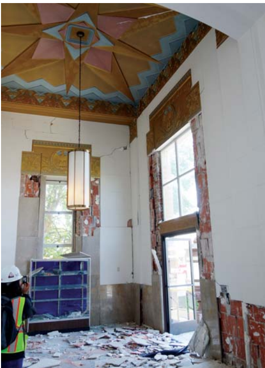
Figure 6. Failing nonstructural elements such as the stone-veneer window and door surrounds shown in this image can become a life-safety hazard when they block or impede an exit path. Photo: Wiss, Janney, Elstner and Associates, Inc.
