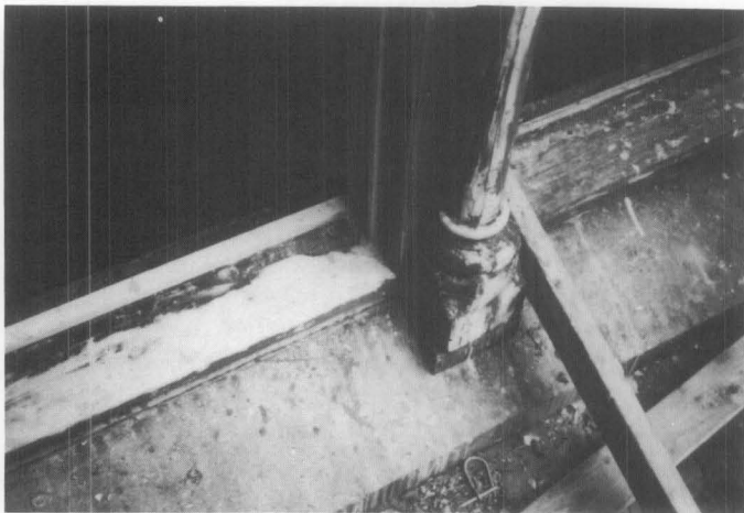
Illus. 7. Whenever possible, historic materials should be repaired rather than replaced. Epoxy, a synthetic resin, has been used to repair the wood window frame and sill at the Auditors Building (1878) Washington, DC. The cured resin is white in this photo and will be primed and painted. Photo: Lee H. Nelson, FAIA.
