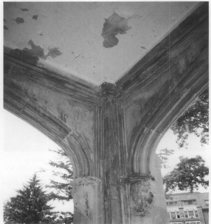
Figure 5. Repeated water washing did not remove the staining inside this limestone porte cochere. Upon closer examination, it was determined to be a water-repellent coating that had been applied many years earlier. An alkaline cleaner may be effective in removing it.
