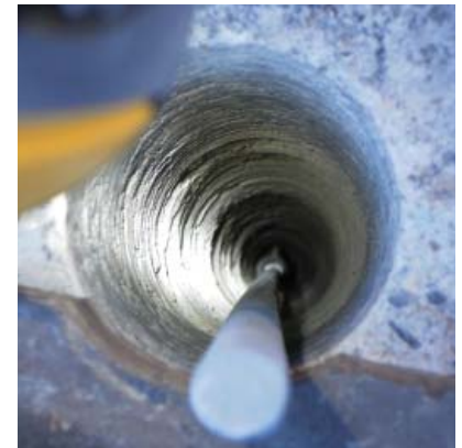
Figure 23. View of one of the center cores drilled down through the wall.
