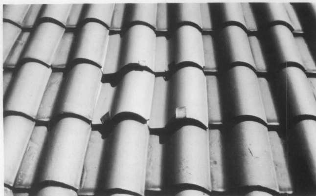
Repairs on this pantile roof were made with new tiles held in place with metal hangers. (Main Building, Ellis Island, New York)
