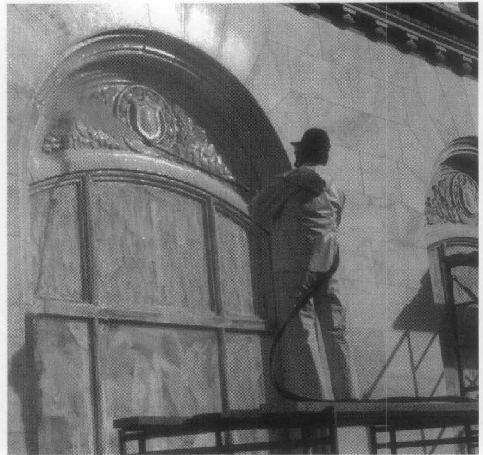
Figure 7. Glazed architectural terra cotta often may be cleaned successfully with a low-pressure water wash and hand scrubbing supplemented, if necessary, with a non-ionic detergent. Photo: National Park Service Files.
