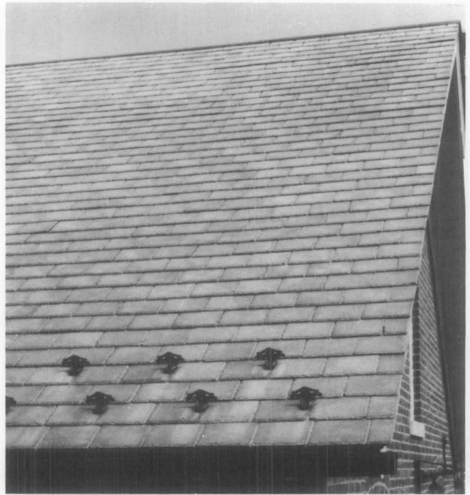
Illus. 14. The visual qualities of the historic feature must be matched when using substitute materials. In this illustration, the lighter weight mineral fiber cement shingles used to replace the deteriorated historic slate roof were detailed to match the color, size, shape and pattern of the original roofing and the historic snow birds were reattached. Photo: Sharon C. Park, AIA.
