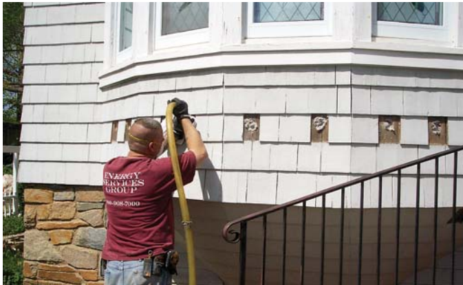
Fig. 18. Dense-packed cellulose insulation is being blown in through holes drilled in the sheathing. Once the operation has been completed, the shingles will be reinstalled. Photo: Edward Minch.
