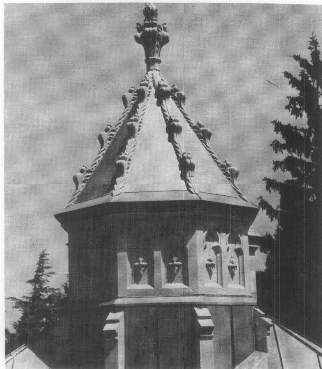
Decorative features such as cupolas require extra maintenance. The flashing is carefully detailed to promote run-off, and the wooden ribbing must be kept well-painted. This roof surface, which was originally tin plate, has been replaced with lead-coated copper for maintenance purposes. (Lyndhurst, Tarrytown, New York, photo courtesy of the National Trust for Historic Preservation)
