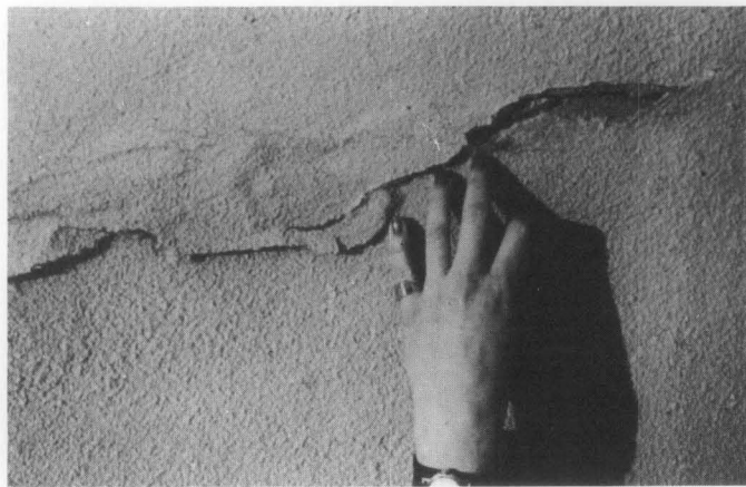
Illus. 6. Substitute materials should never be considered as a cosmetic cover-up for they can cause great physical damage and can alter the appearance of historic buildings. For example, a fiberglass coating was used at Ranchos de Taos, NM, in place of the historic adobe coating which had deteriorated. The waterproof coating sealed moisture in the walls and caused the spalling shown. It was subsequently removed and the walls were properly repaired with adobe. Photo: Lee H. Nelson, FAIA.
