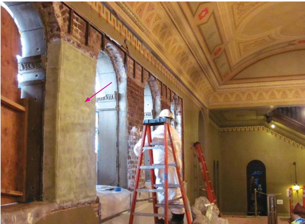
Figure 26. Epoxy-embedded fiberglass mesh is being bonded to the back of the brick pilasters of this 1906 unreinforced masonry building. New finishes matching the appearance and detailing of the original finishes will be applied over the mesh. Photo: Wiss, Janney, Elstner and Associates, Inc.
