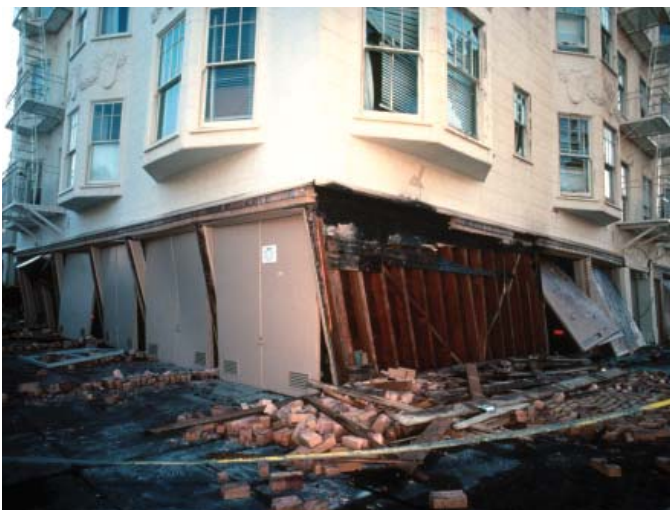
Figure 30. Large perimeter openings and a limited number of interior partitions on the ground floor can create a “weak story” condition that makes buildings particularly vulnerable to earthquake damage. Photo: USGS.
