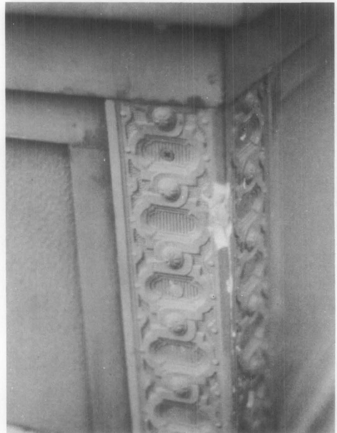
Illus. 20. Long-term performance can be affected by where the substitute material is located. In this case, fiberglass was used as part of a storefront at street level. Due to the brittle nature of the material and the frequency of impact likely to occur at this location, an unsightly chip has resulted. Photo: Sharon C. Park, AIA.
