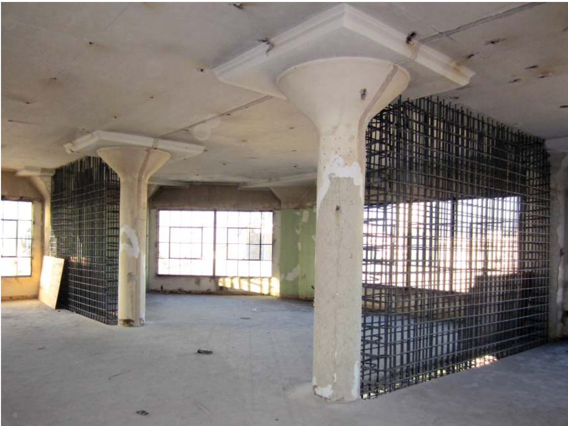
Figure 28. Steel reinforcement for the new shear walls, perpendicular to the windows, is being installed in this concrete-frame building. Photo: Robert Chattel.
