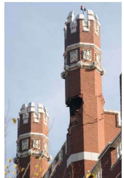
Figure 1. In 2011, a 5.6 magnitude earthquake substantially damaged all four turrets atop St. Gregory's University Benedictine Hall in Shawnee, Oklahoma. Photo: St. Gregory University.
