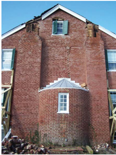
Figure 19. Chimneys are common nonstructural features susceptible to earthquake damage, even in zones of low-to medium-seismic activity as shown on this building in Virginia damaged in a 2011 earthquake. Photo: Suzanne Tripp.
