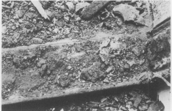
Fig. 6 d. View looking down towards the sill. The subframes appeared very rusted, but were in good condition once debris was vacuumed and surface rust was removed, in place, with chemical compounds. Where necessary, epoxy and steel filler was used to patch depressions in order to make the subframe serviceable again.
