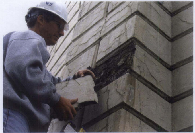
Figures 14. Layers of architectural concrete that have debonded (spalled) from the surface were removed from a historic water tank during the investigation performed to assess existing conditions. Photos: Anita Washko, Wiss, Janney, Elstner Associates, Inc.
