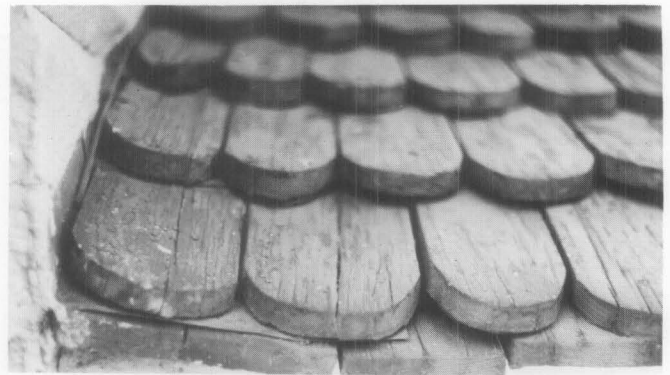
Replacement of particular historic details is important to the individual historic character of a roof, such as the treatment at the eaves of this rounded butt wood shingle roof. Also note that the surface of the roof was carefully sloped to drain water away from the side of the dormer. In the restoration, this function was augmented with the addition of carefully concealed modern metal flashing. (Mount Vernon, Virginia)
