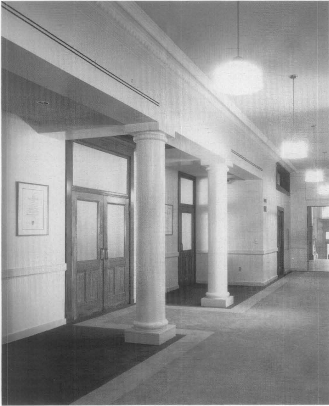
b. Central air conditioning was installed in the corridors of this circa 1900 school building by adding an air handler over the entrance from a vestibule. The custom-designed slot registers provide linear diffusers without detracting from the architecture of the space. Photo: Lautman Photography courtesy of Notter Finegold + Alexander Inc.
