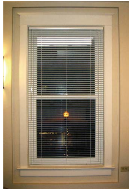
Fig. 20. The walls have been furred out inappropriately around the historic window trim creating an appearance the interior never had historically.
