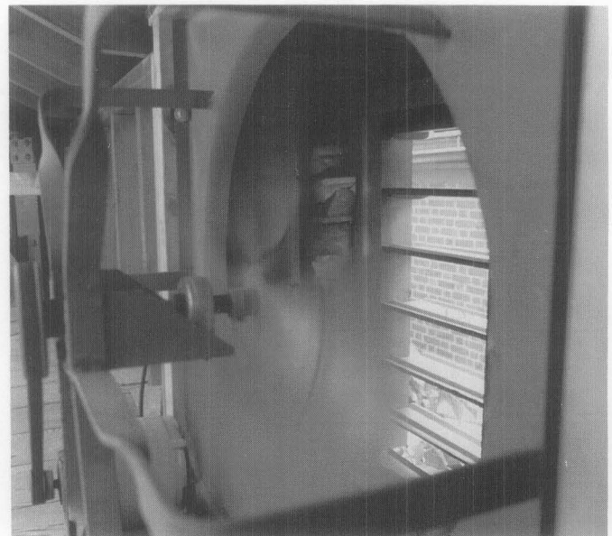
9. Improving ventilation through traditional means should not be overlooked in planning new or upgraded HVAC systems. In mild climates, good exhaust fans can often eliminate the need for air conditioning or can reduce equipment size by reducing cooling loads. Photo: Ernest A. Conrad, P.E.
