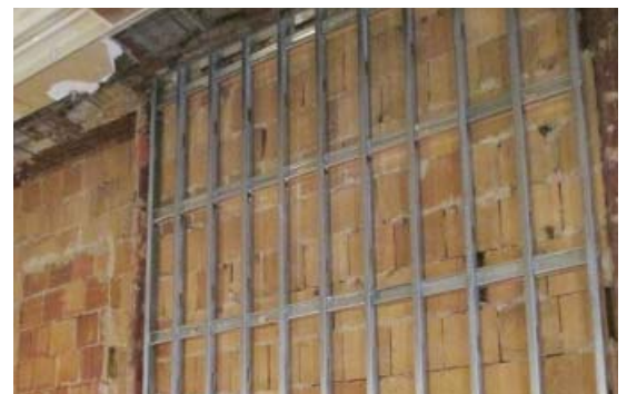
Figure 27. A new steel stud wall is being added to one side of this interior hollow-clay tile wall. The side with the least amount of historic finishes was chosen as the least disruptive location for the added reinforcement. The wall will be returned to its original appearance by installing new finishes matching the historic finishes. Photo: Wiss, Janney, Elstner and Associates, Inc.
