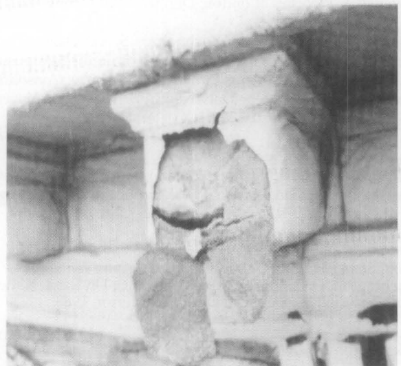
Figure 27. Instead of correcting the roof drainage problems, an elastomeric coating was applied to the already saturated limestone cornice. An elastomeric coating holds moisture in the masonry because it does not "breathe" and does not allow liquid moisture to escape. If the water pressure builds up sufficiently it can cause the coating to break and pop off as shown in this example, often pulling pieces of the masonry with it. Photo: National Park Service Files.
