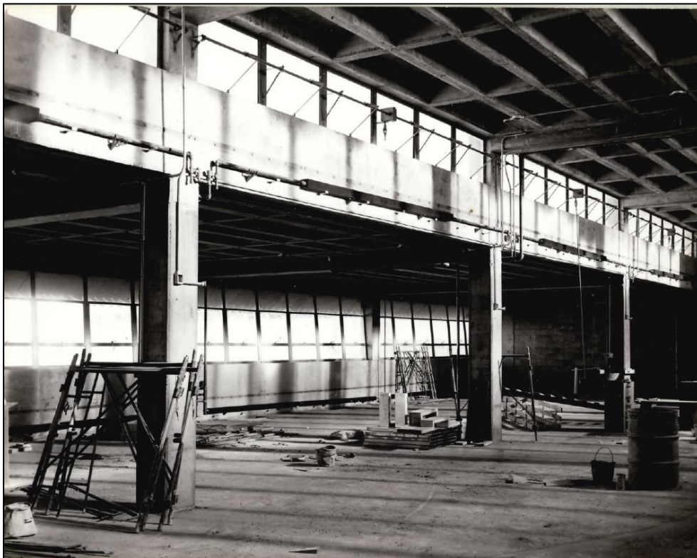
Figure 2-56. Interior of Room 358, Wing 3, under Construction, November 30, 1953 (photograph courtesy of Department of Commerce Boulder Laboratories)
