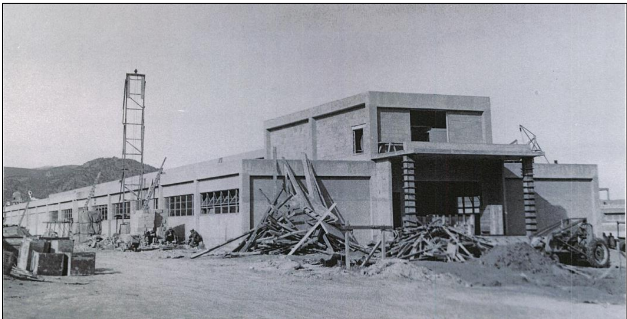
Figure 2-8. Wing 6 under Construction circa 1956, view north (photograph courtesy of Carnegie Library for Local History, Boulder, Colorado, Chamber of Commerce Collection)
