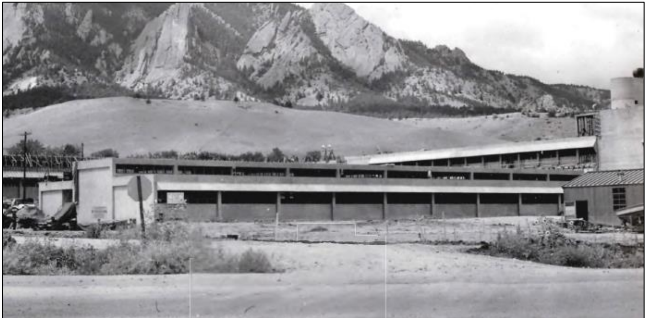
Figure 2-28. East and North Elevations of Wing 2 under Construction, July 31, 1953 (view west; cropped and enlarged to show detail; annotations added by SDC and AECOM; photograph courtesy of Department of Commerce Boulder Laboratories)
