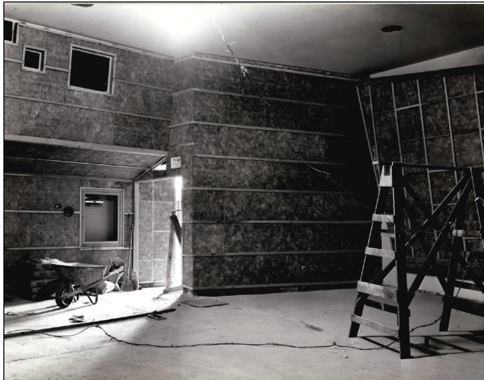
Figure 2-46. South and West Walls of Auditorium under Construction on January 31, 1954 (photograph courtesy of Department of Commerce Boulder Laboratories)
