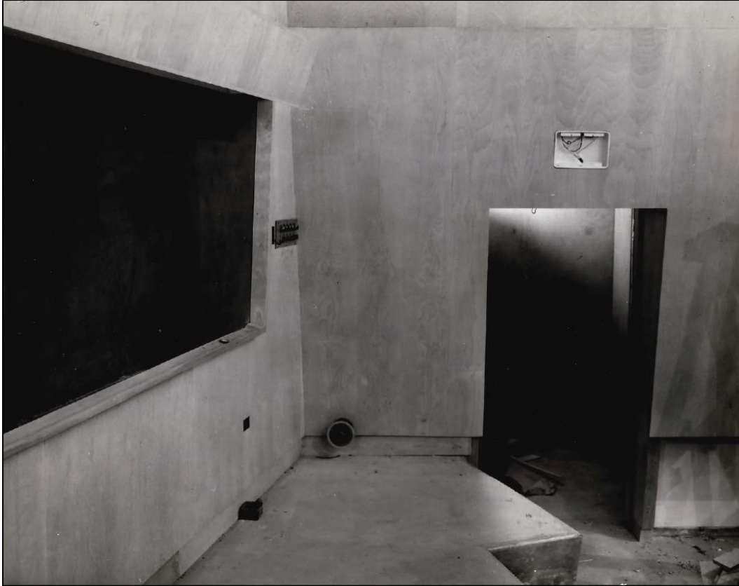
Figure 2-48. Stage and West Stage Door under Construction on March 31, 1954 (photograph courtesy of Department of Commerce Boulder Laboratories)
