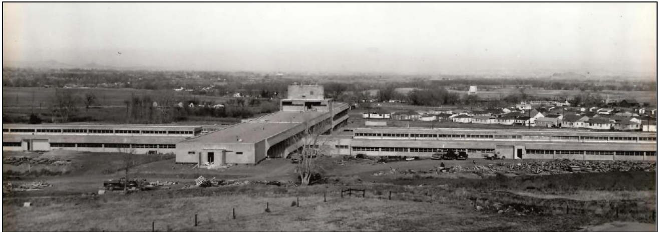
Figure 2-16. South End of the Spine under Construction, November 30, 1953 (view northeast; photograph courtesy of Department of Commerce Boulder Laboratories)
