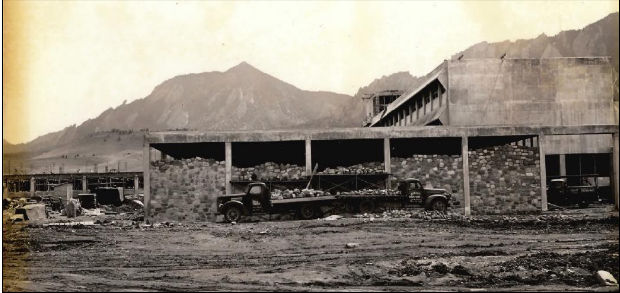
Figure 2-20. North Elevation of the Library at the Front of the House under Construction, June 2, 1953 (view southwest; photograph courtesy of Department of Commerce Boulder Laboratories)
