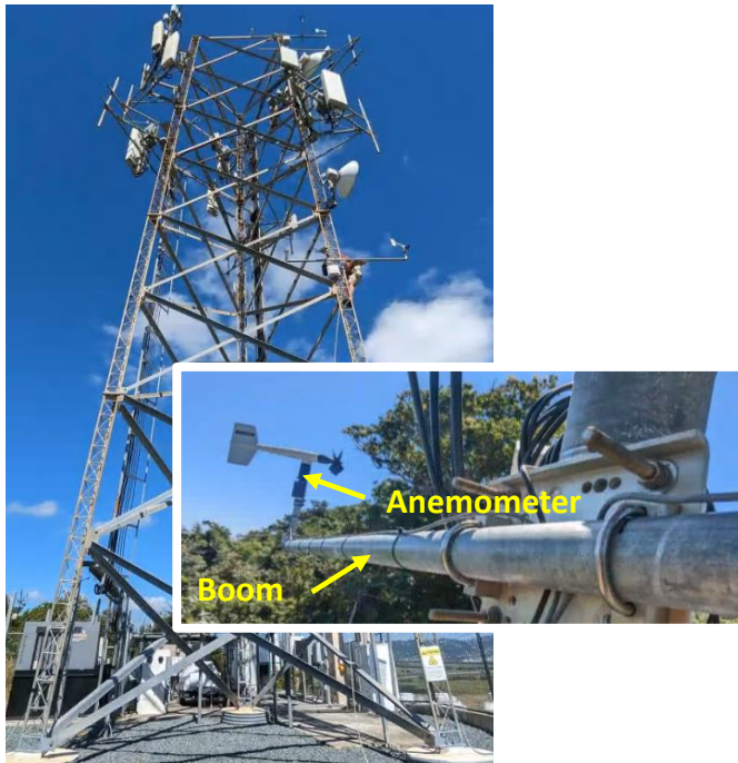
Anemometers as installed on YTA tower
