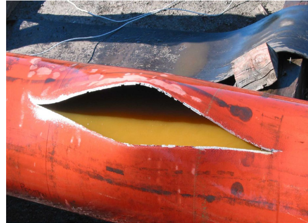
Rupture after hydrotesting
