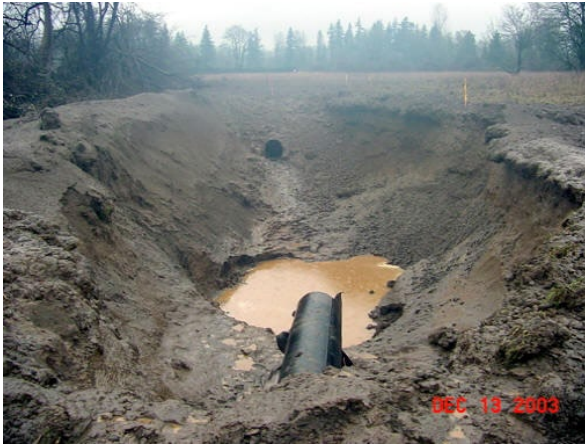
Blowout of a gas pipeline
