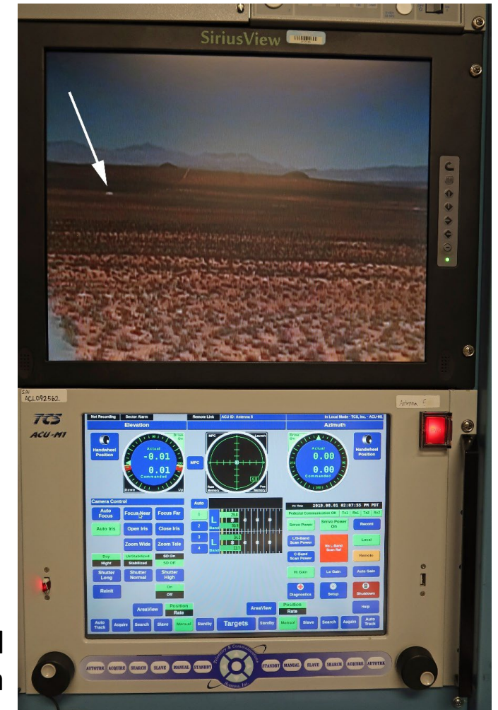
Antenna Control and Camera
