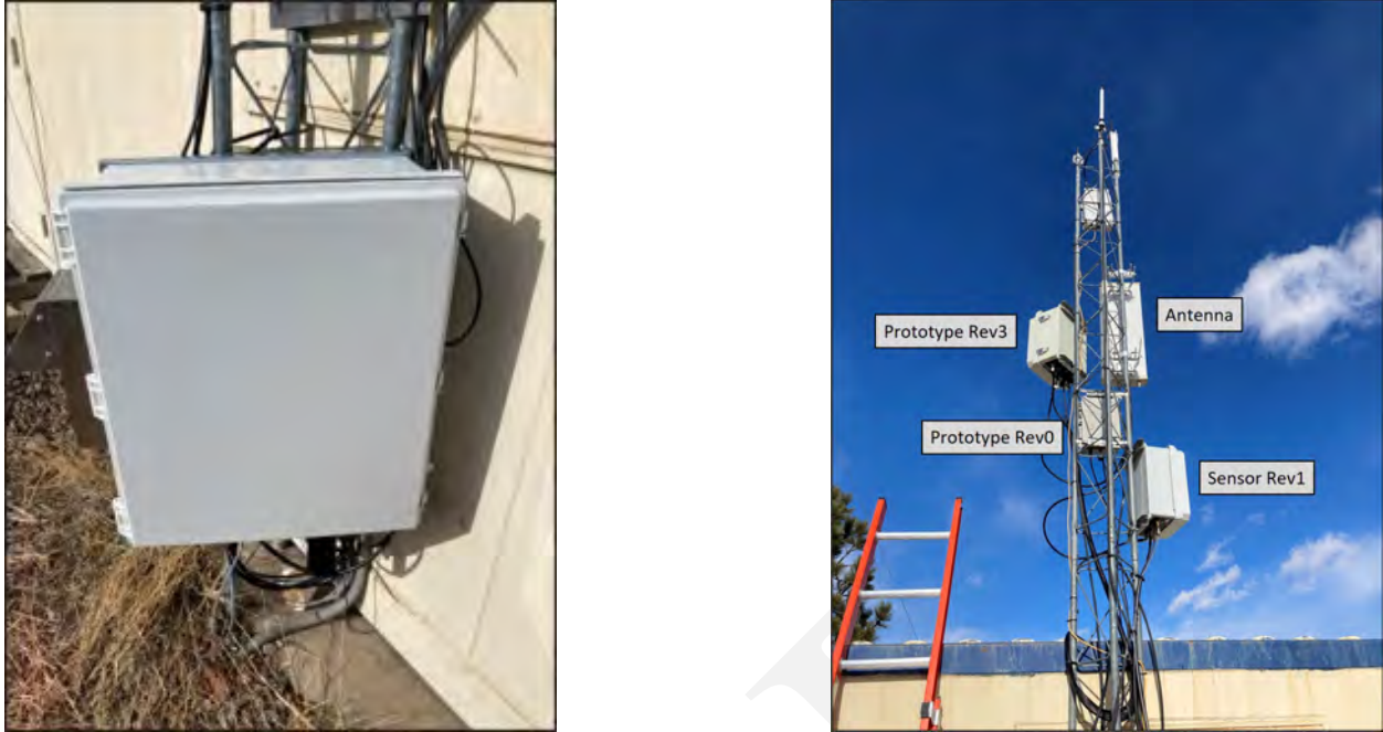
Figure 6.1: Installation of the new sensor design at GMM with the SPU (left) and preselector (right). Note the preselectors for other sensor revisions are located near the sensor revision 1 preselector as well.
