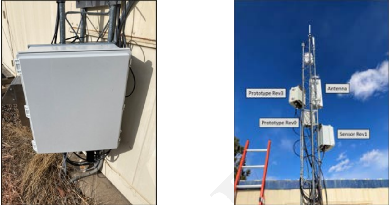
Figure 6.1: Installation of the new sensor design at GMM with the SPU (left) and preselector (right). Note the preselectors for other sensor revisions are located near the sensor revision 1 preselector as well.
