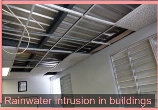
Building envelope damage
