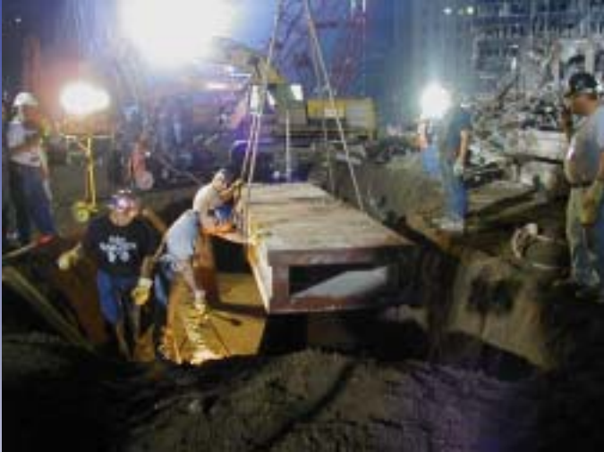
Clean weld fracture of Interior columns
