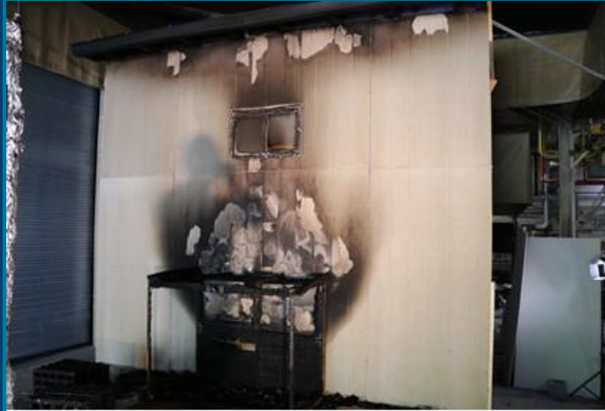
Significant spalling of cement board
