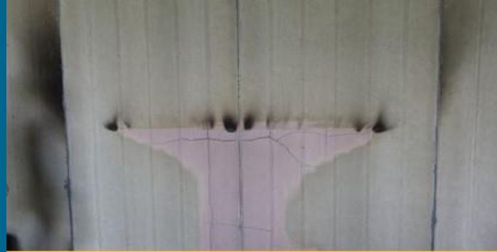
Cracking of cement board
