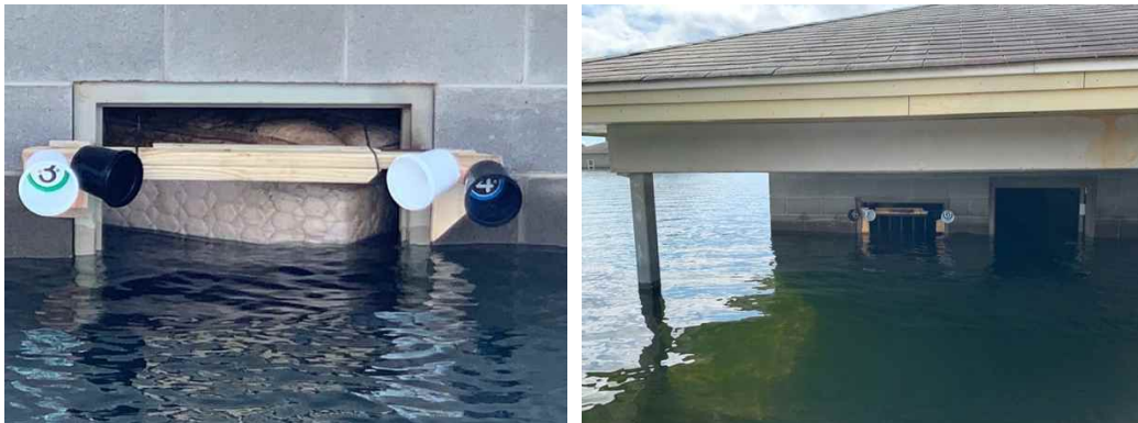
Figure 31) LEFT: Other inspection tasks required the drone to hover low above the water to look in windows and doors. The two positions and orientations designated by the white and black pairs of buckets guided the pilot to completely inspect the floating mattress looking for survivors (visual or thermal). RIGHT: Similar window inspection tasks were located under a more difficult covered porch near a door. That's where underwater versions of these same tests were embedded for underwater system reconnaissance.
