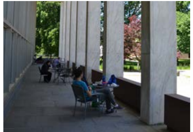
There is an alternating pattern between the columns and the barrier wall
