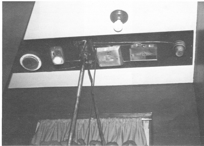
Detector Placement — Head of Basement Stairs (Whitehouse)
